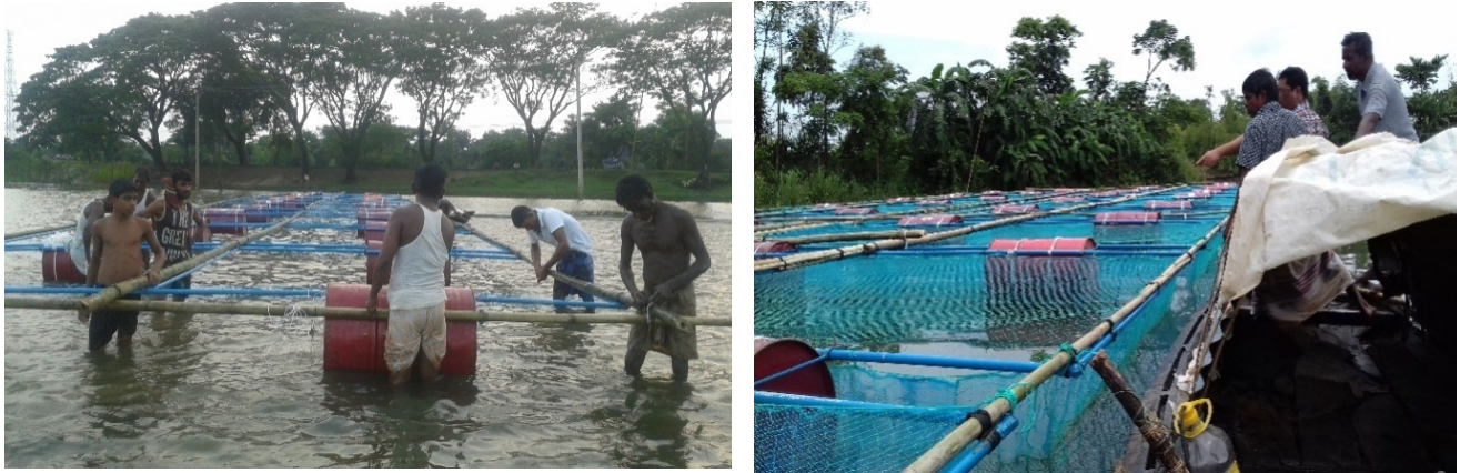
Plate 2: Construction of cage frame by GI pipe, bamboo and other materials (left) and PI observed the cage unit in the haor floodplain after setting cage frame (right)
