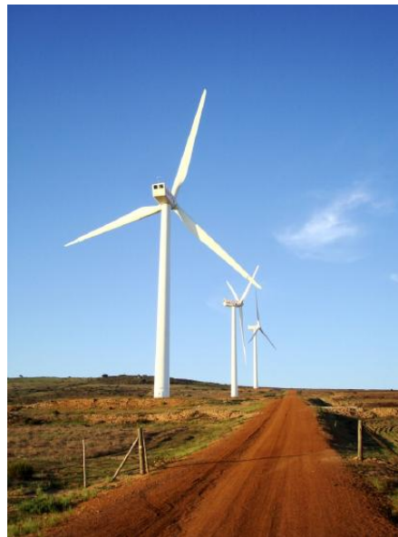
Figure 6.7.1: GE combines environmental responsibility with the business strategy of providing the best wind energy devices. warrenski – Darling Wind Farm – CC BY-NA 2.0.
