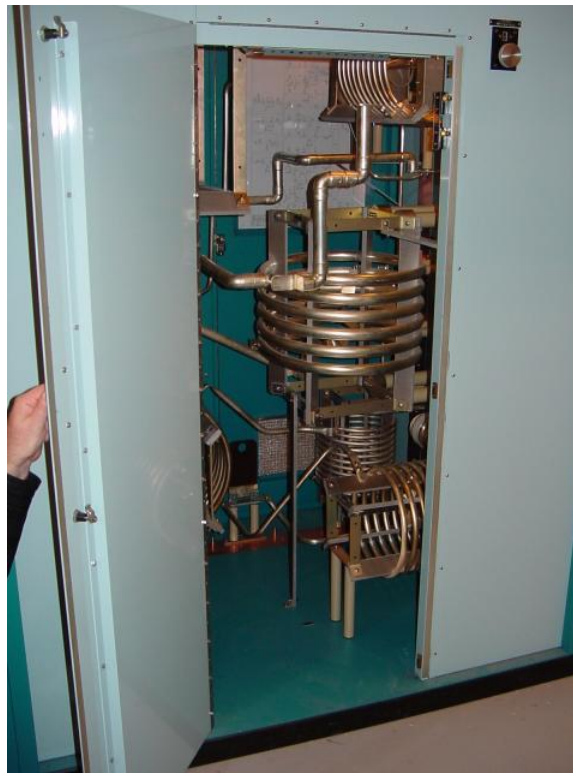
High power inductors formed from hollow tubes.
