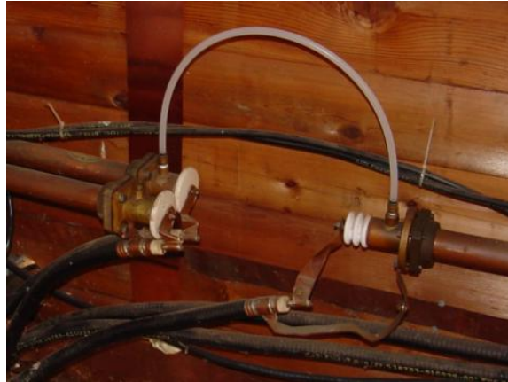
Flexible coaxial cables connected to rigid lines.
