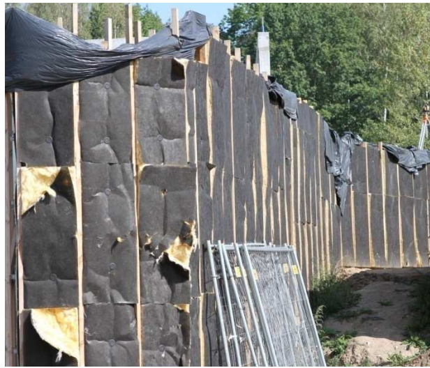
Fig. 1. New building insulated with mineral wool panels not protected against wind-washing
