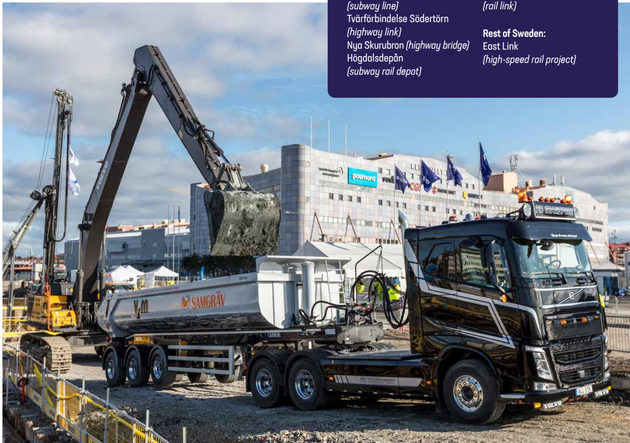
→ VSM and Samgräv have been contracted on excavation and haulage respectively on the Västlänken infrastructure project.
