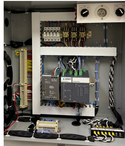
New Low Voltage Compartment
