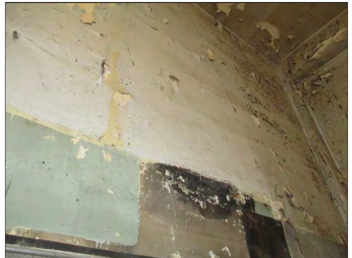
10. Suspect mold growth in the storage room wall
