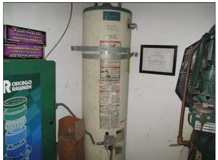
24. Electric hot water heater
