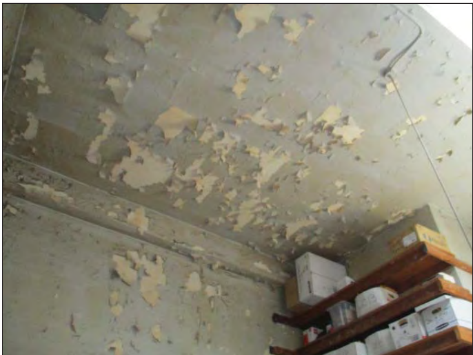
9. Chipped/peeling paint in the storage room walls and ceilings
