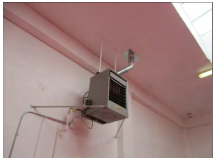
34. Natural gas space heater
