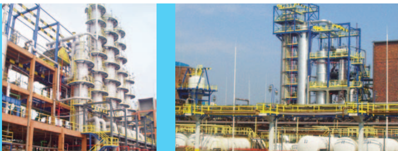
Ethyl-benzene plant, Petrochemia Blachownia
