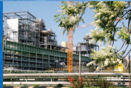
Waste water evaporator and crystallizer plant section
