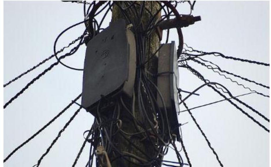
Aging BT Openreach infrastructure
