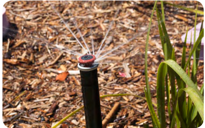
Multi-stream nozzles throw streams of water with larger water droplets which help to prevent misting and runoff. Each nozzle should be checked periodically to be sure it is operating correctly.
