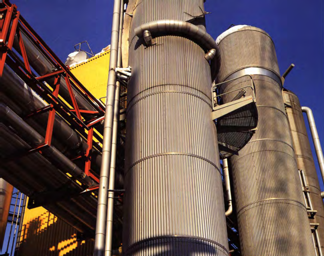
Akzo Nobel's hydrogen peroxide plant, Bohus, Sweden
