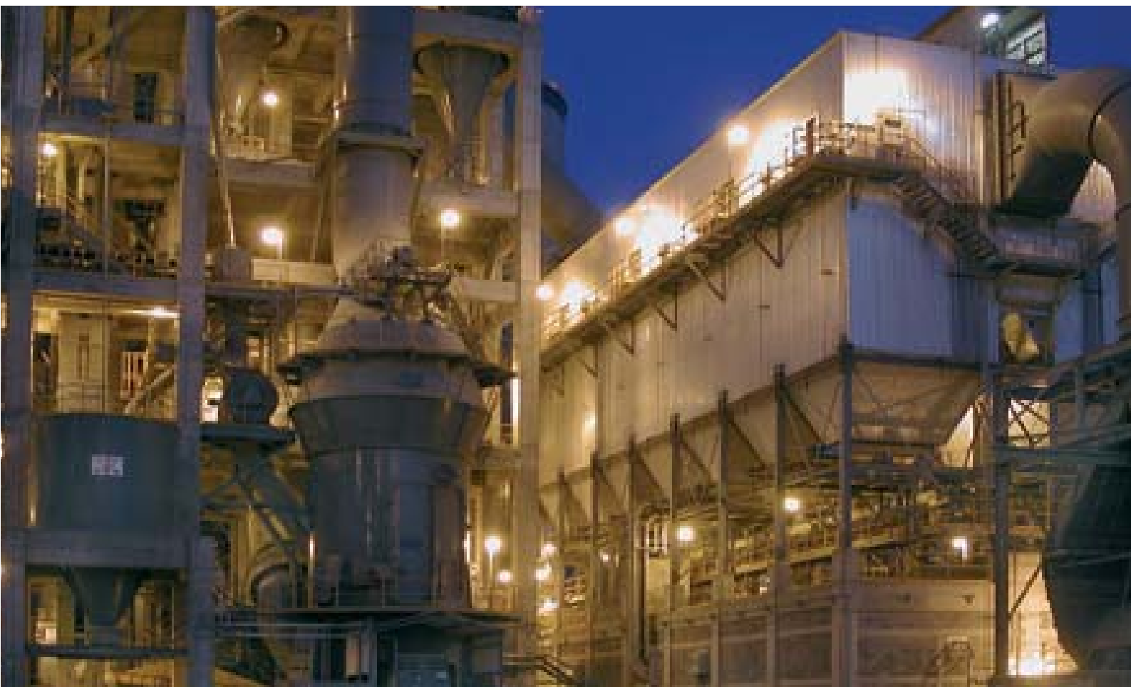
Raw mill and bag filter at Holcim Apasco's Ramos Arizpe plant in Mexico.
