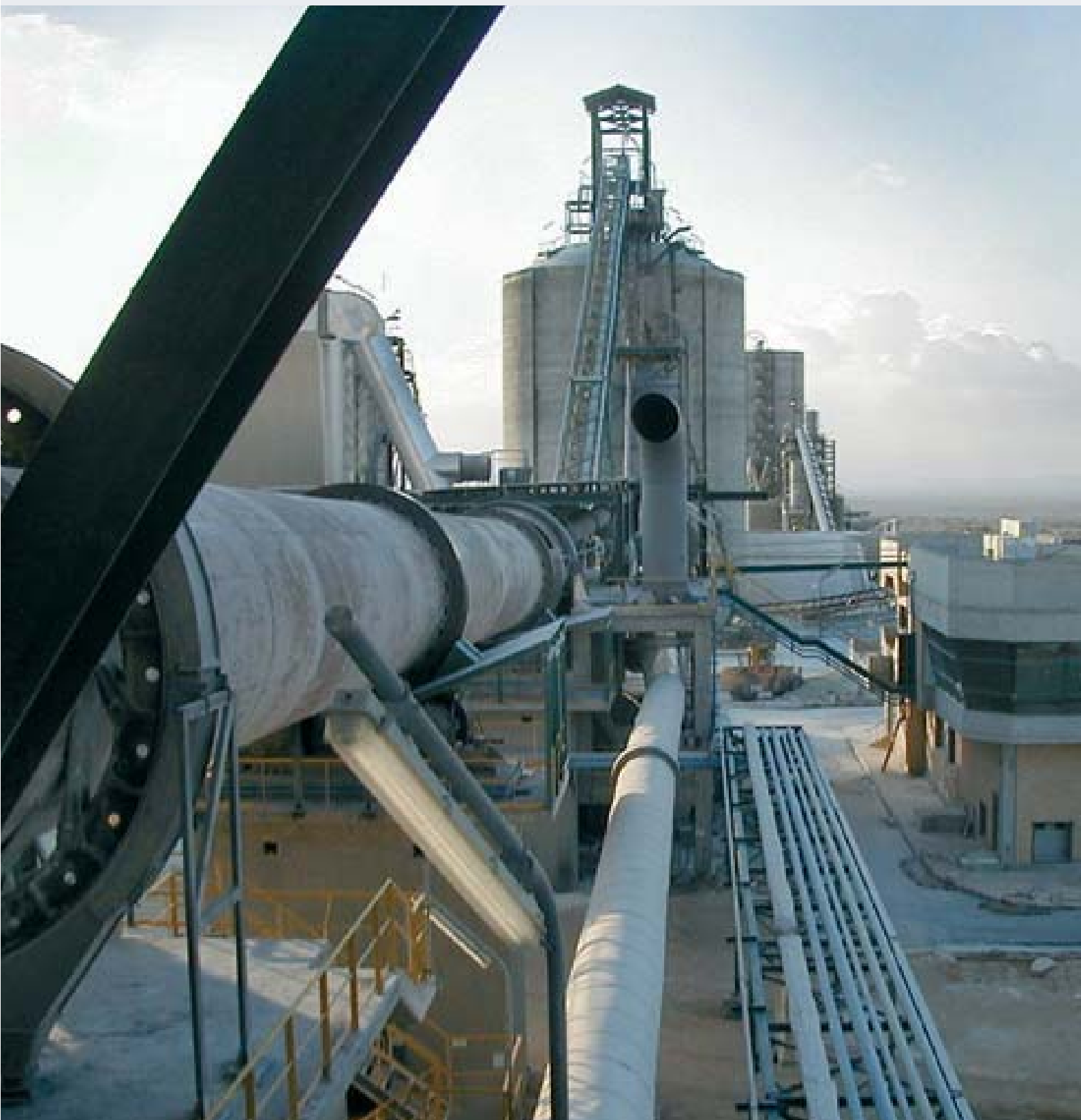
The rotary kiln at Sinai White Portland Cement, which is owned by Aalborg Portland, produces more than 1000 tonnes white cement per day.
