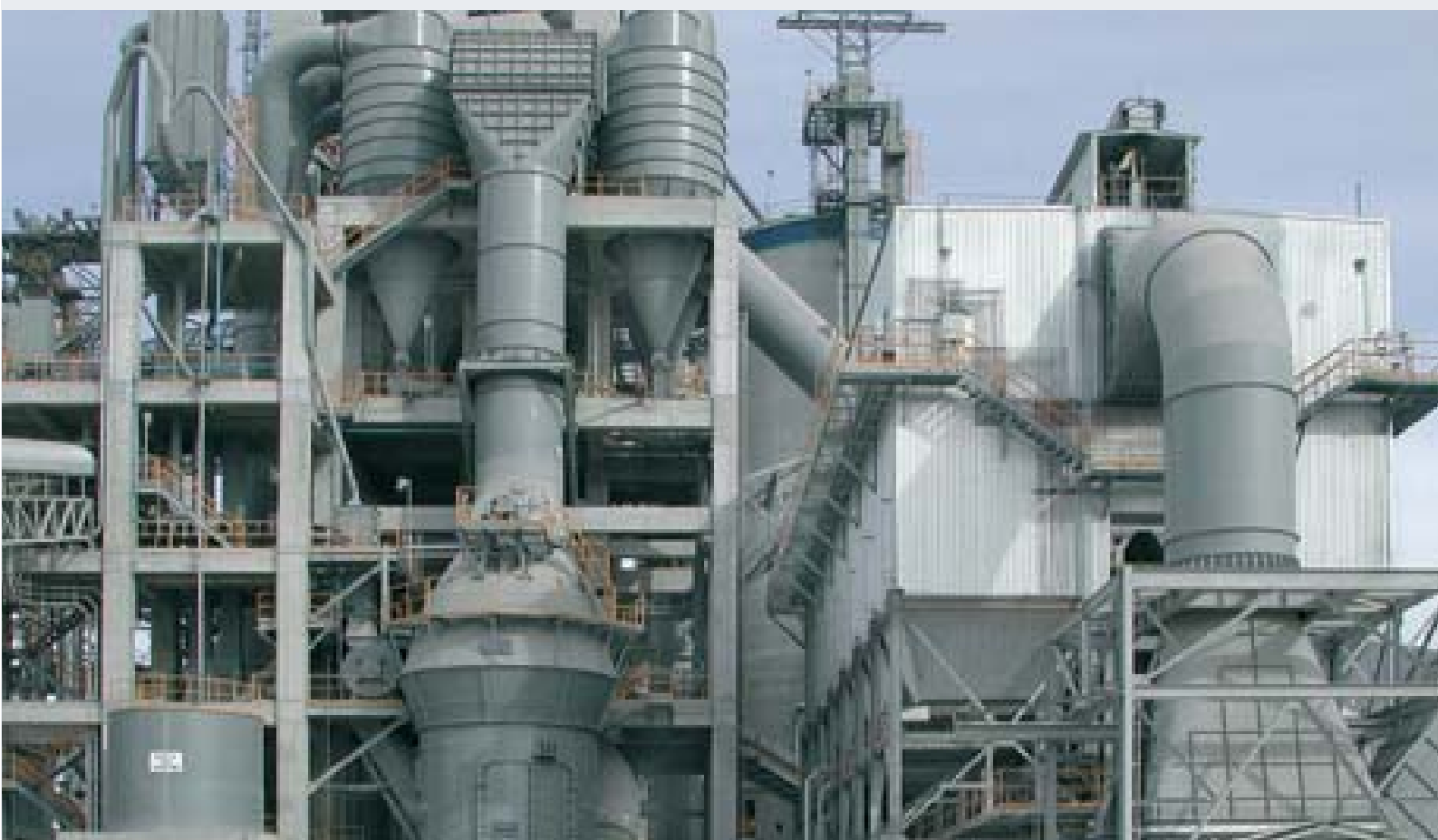
F.L.Smith supplied this ATOX raw mill to the Ramos Arizpe plant in Mexico.
