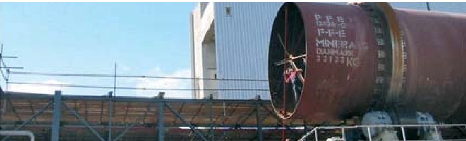
Lime reburning kiln supplied by FFE Minerals being erected at the Zellstoff Stendal pulp mill in Germany.
