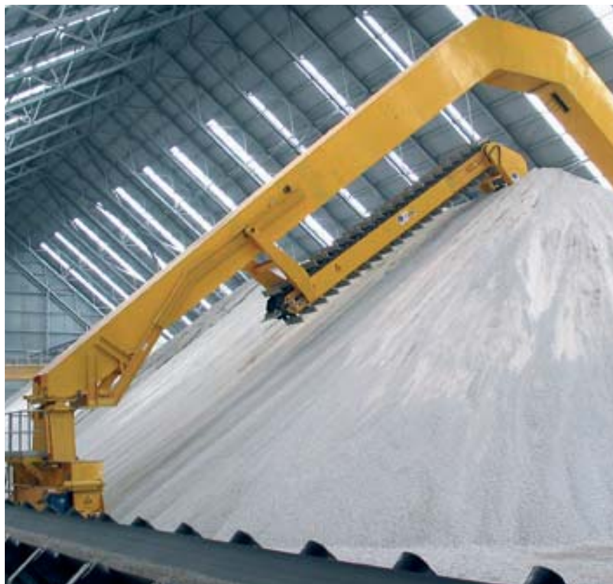
F.L.Smidth Materials Handling supplied this limestone storage for the West Burton power station in the UK.
