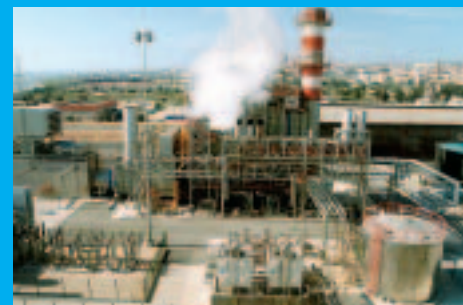
6. Cogeneration at Povia (P)
