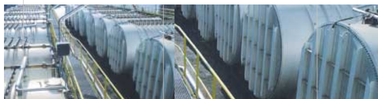
Seawater desalination plants with stainless steel heat exchangers
