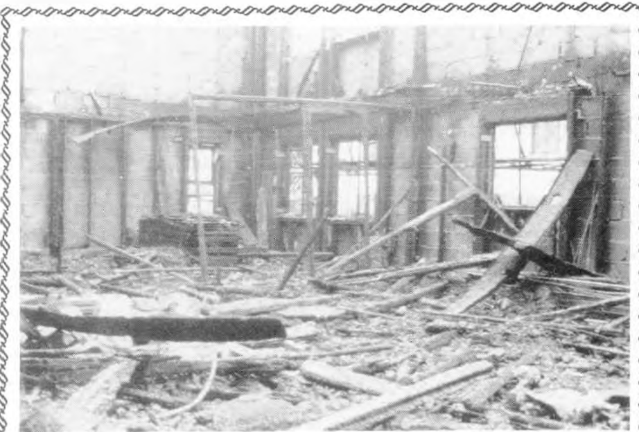
Fire damage on £160,000 houses at Beechwood Rise, Tromode.
