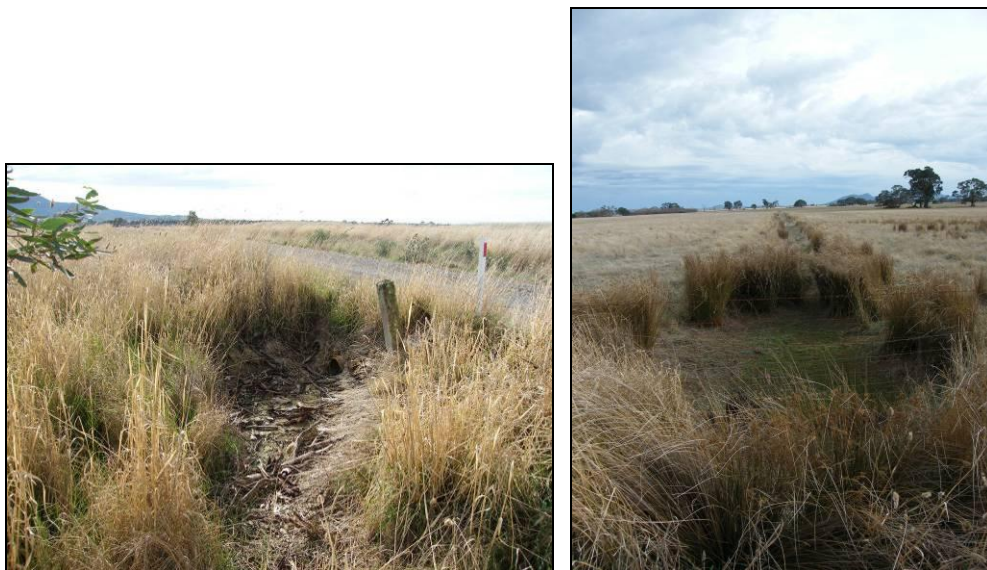
Site 12. Middle Creek tributary at Western Highway – north (left) and south (right).
