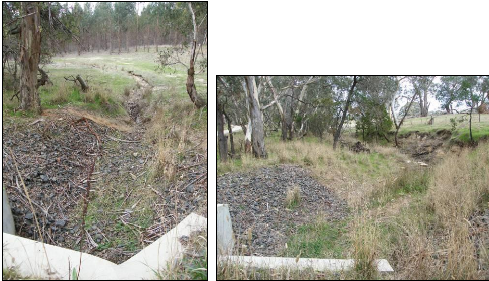
Site 22. Billy Billy Creek tributary at Peacocks Road – west (left) and east (right).
