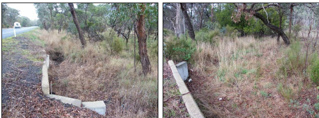
Site 30. Billy Billy Creek tributary at Western Highway – north (left) and south (right).
