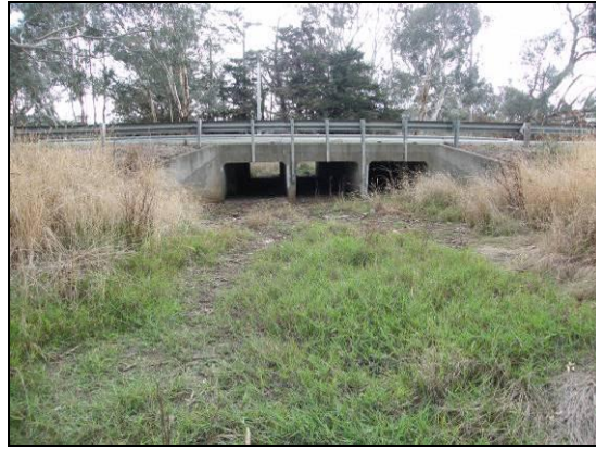
Site 16. Charliecombe Creek tributary at Western Highway – north (left) and south (right).
