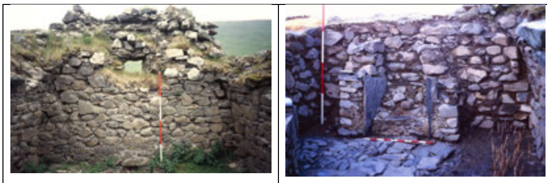
Plates 8 & 9 showing the curvature of the vault, slit window, later fireplace and floor stakes. Note the gable walls are not bonded into the long walls.
