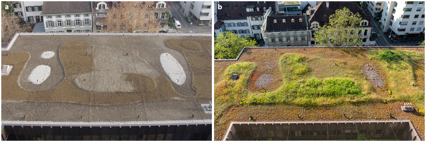
Fig. 1: Green roof of the University Hospital Basel, Klinikum 2. The pictures show a diverse substrate composition and varying thickness thereof. a. after installation in 2003 (Photo: Stephan Brenneisen); b. how vegetation composition is adapting to the different habitat conditions over the years. The picture was taken in 2021 (Photo: Andreas Hofstetter)
