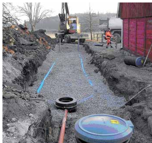
Small-scale infiltration plant for sewage treatment.
