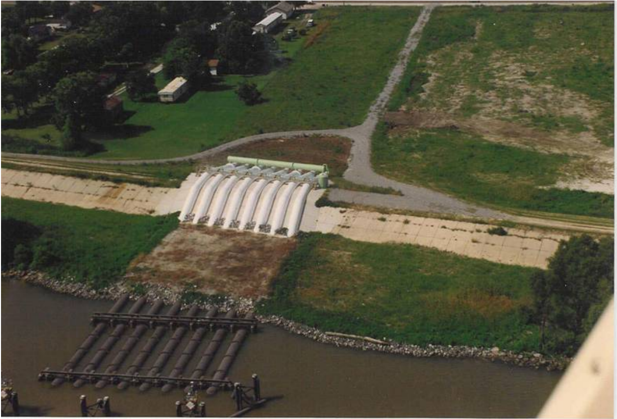
Figure 1. The West Pointe a la Hache siphons (BA-04) were constructed in 1992 and funded by the state of Louisiana. Mississippi River water was siphoned from the river intakes, discharged into a ponding area, and distributed through four channels into the surrounding marshes.
