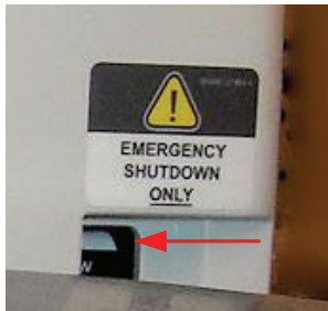
Figure 10-6: Breaker Position OFF
