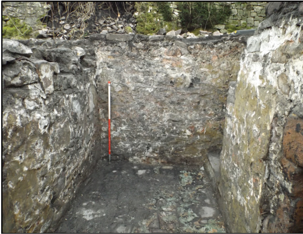
Plate 1. East-facing elevation of front (west) wall leading to staircase to the right (view west)
