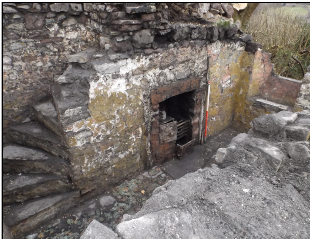
Plate 20. Chimney breast and staircase, incorporated into northern gable end wall (view northeast)
