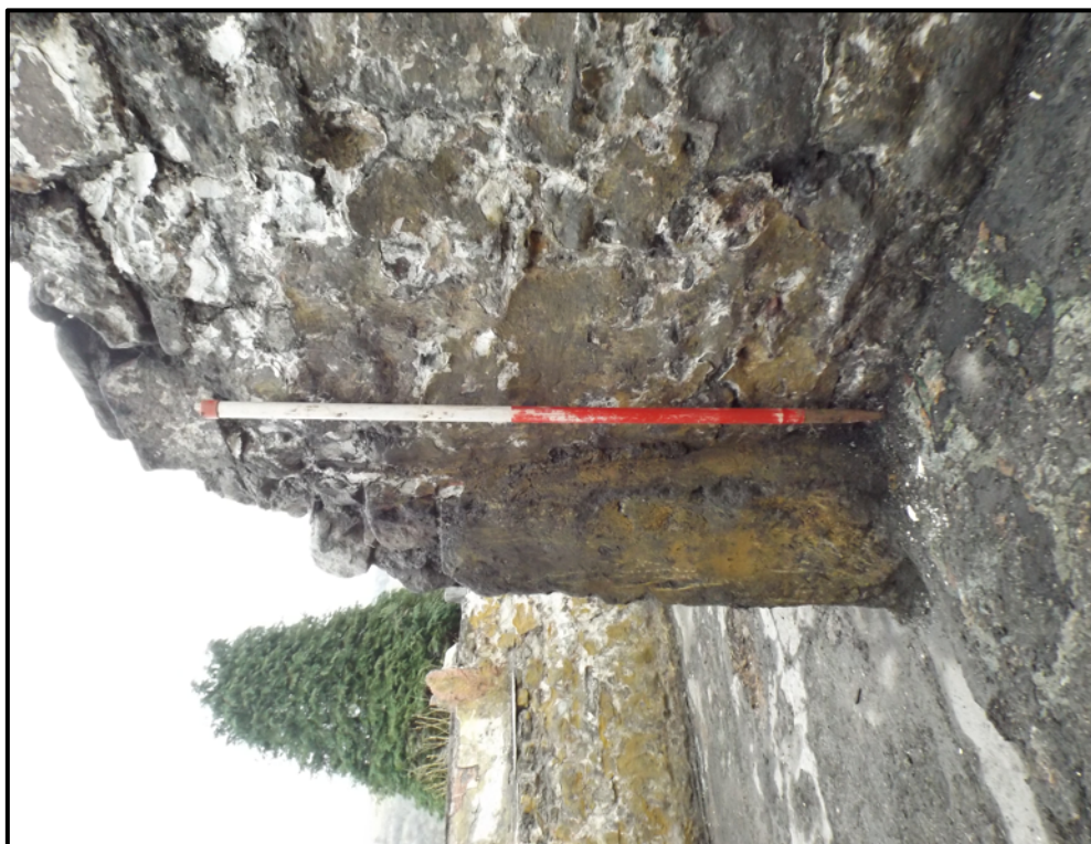
Plate 6. Protruding section of masonry at juncture between primary and secondary partition walls (view southeast)
