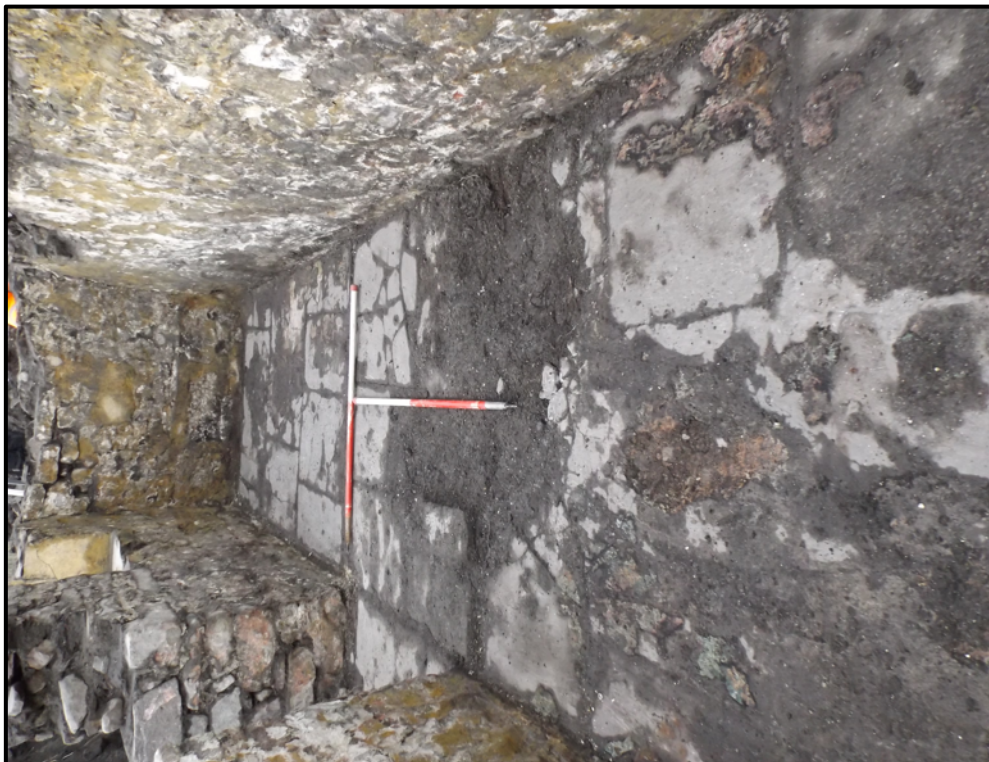
Plate 22. Remains of flagstone flooring with some remnant linoleum and bitumen to west of rear doorway (view south)
