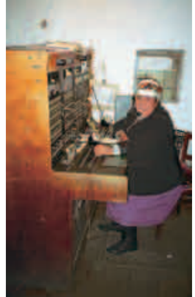
Switchboard in Murgab, serving an area the size of Switzerland. Although over 50 years old, the switchboard is still functioning. However, its reliability and transmission quality are rapidly decreasing and do not even meet minimal standards. (Photo: A. Haslinger)
