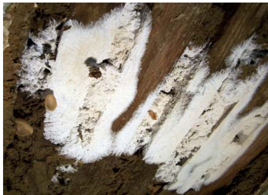
Photo 6 – The rapid expansion of mycelium of Peziza domiciliana Cooke in the floor, historical house, Stefan cel Mare Street, 75, Targu Neamt
