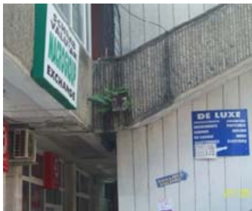
Fig. 4. Fern development on the Cluj-Napoca building wall, May, 2009
