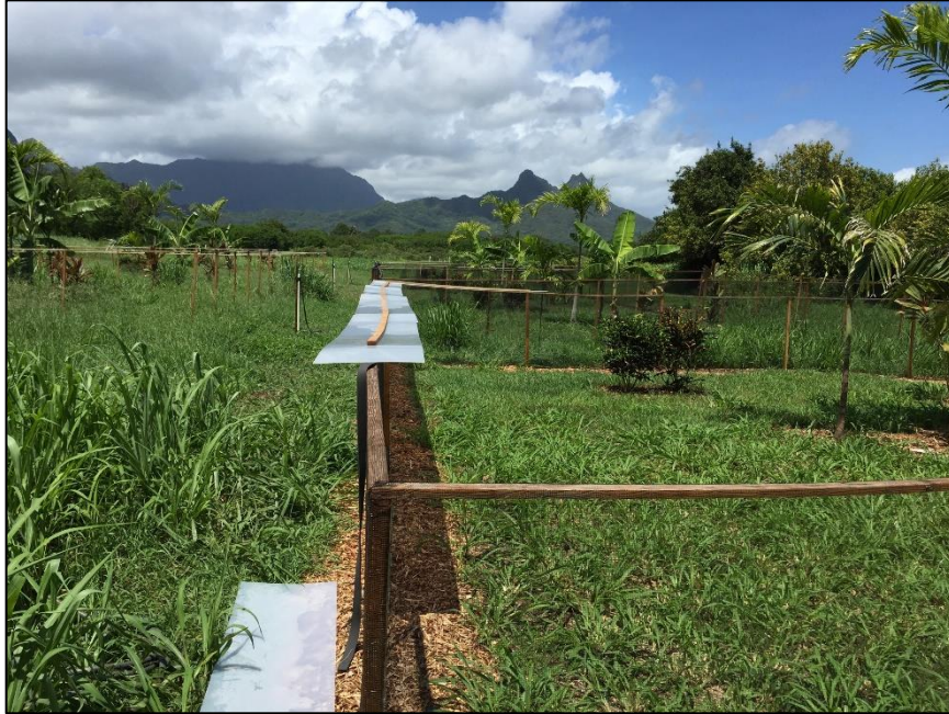
Figure 3. Hawaii enclosures, installing top plastic in progress. The wooden frame is in place (2x2" uprights, 1x2" top frame), and the mesh is stapled to the frame on top and buried on the bottom. The black gasket material (1/4" thick neoprene) can be seen draping off to the left. The top of the enclosure is a sandwich of 1x2" wood, gasket, plastic, 1x2" wood, all screwed together. The plastic lip
