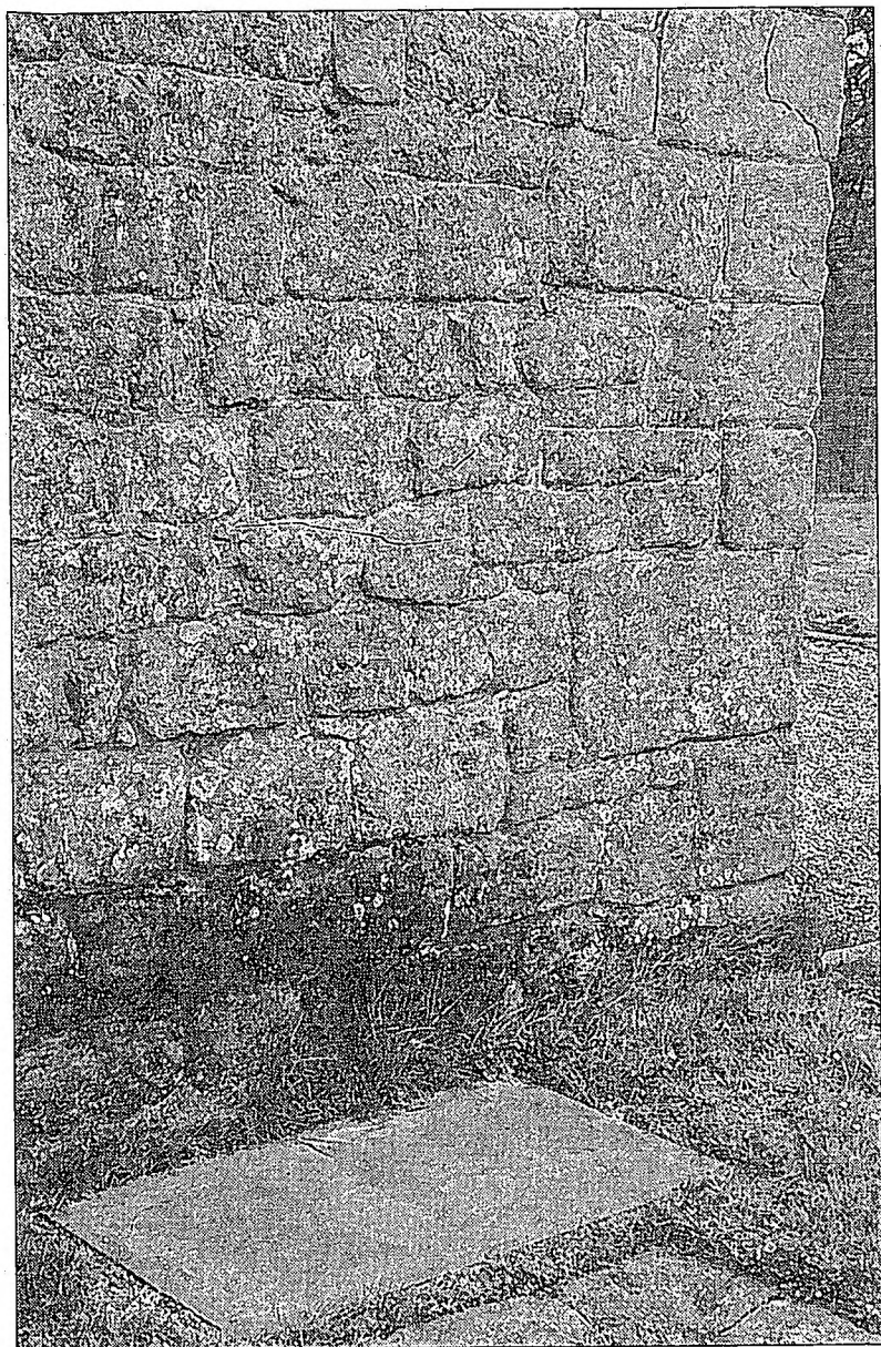
Fig. 2. The base tower before (upper) and after (lower) the replacement of the stone slab. The stone-ringed drain is visible in the foreground.
