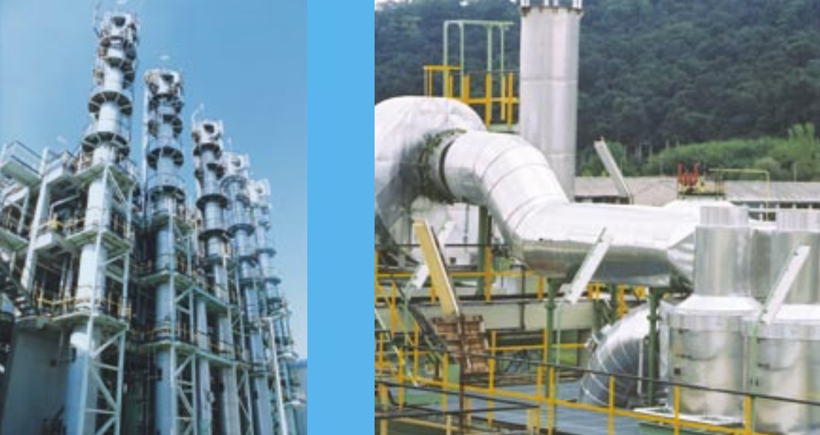
Vinyl-chloride extraction columns
