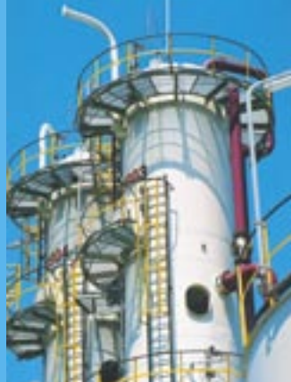
View of TDI Plant
