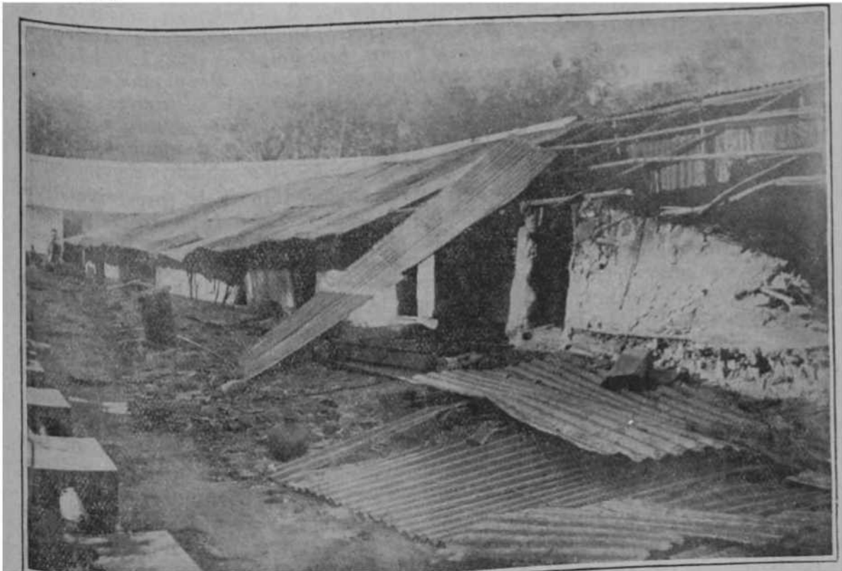
PORTION OF ONE OF THE WINGS OF THE OLD COOLIE QUARTERS JUST DEMOLISHED IN THE FOREGROUND AND PORTIONS OF ONE OF THE BLOCKS OF THE NEW COOLIE QUARTERS IN THE BACKGROUND.
