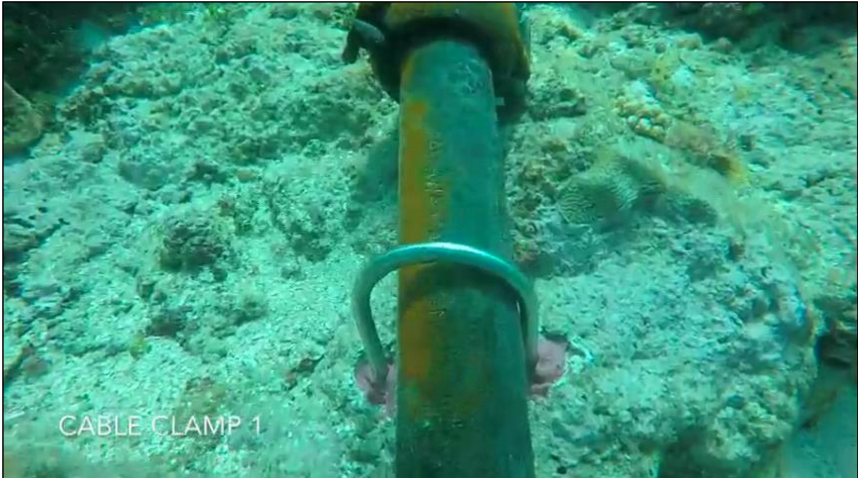
Photo 4. Cable pin installed on the ATISA Cable in 2017. The same hardware and methods would be used for the HK-G Cable pin installation.
