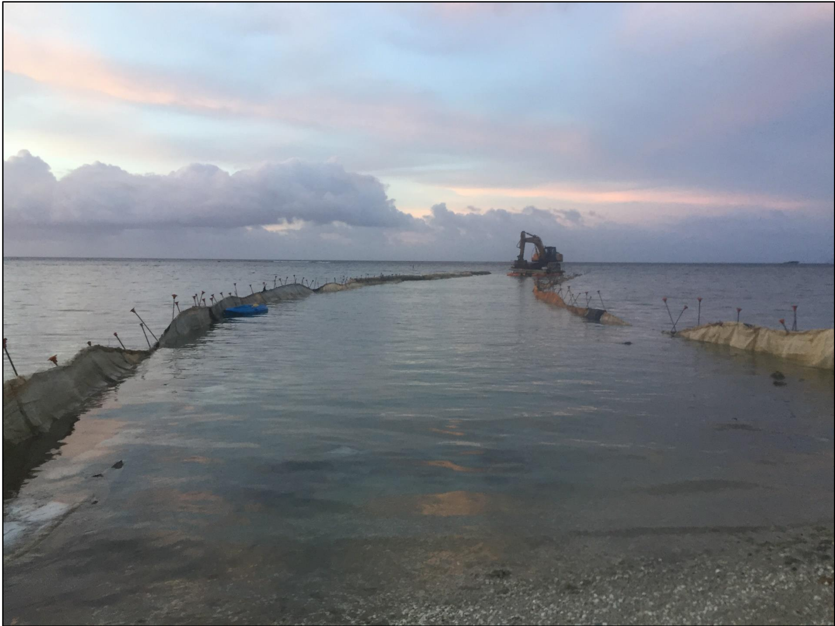
Photo 3. GTA conduit raceway construction corridor. The entrance corridor to allow for small support vessels and pedestrian access would be located entirely within this corridor and would have a smaller area.
