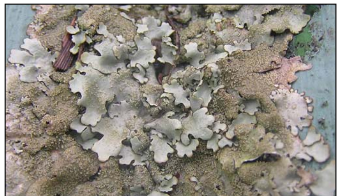
Figure 3. Xanthoparmelia scabrosa on a painted corrugated iron roof, Mangere Bridge. Note the abundant, granular isidia
