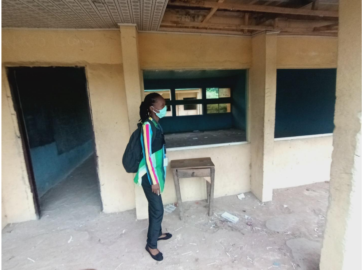
Figure 3: Vandalized classroom at Umuriam Technical School, Obowo
