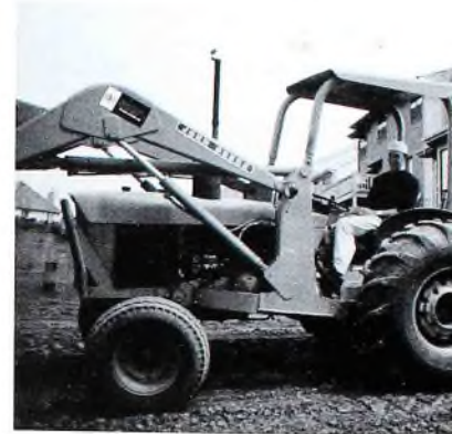
After a hard week of school, senior Matt Waller helps his dad build their new house. Nearly three-fourths of the student body had some type of part-time job. (photo by Jennifer Paskach)
