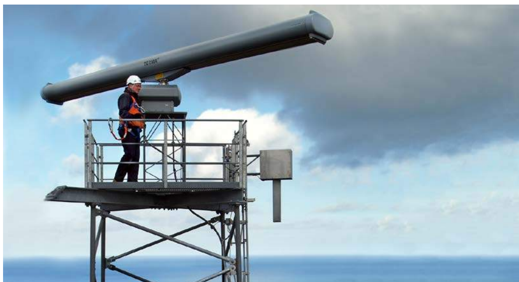
Figure 2.1 Typical antenna installation
