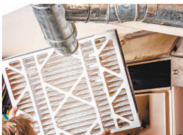
CHARLES KNOWLES TNS Keeping filters up to date is a vital part of HVAC maintenance. Collected dust impedes air flow.
