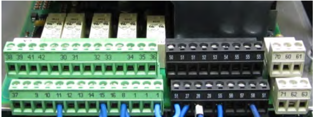
Figure 8-13 Control cable terminals
