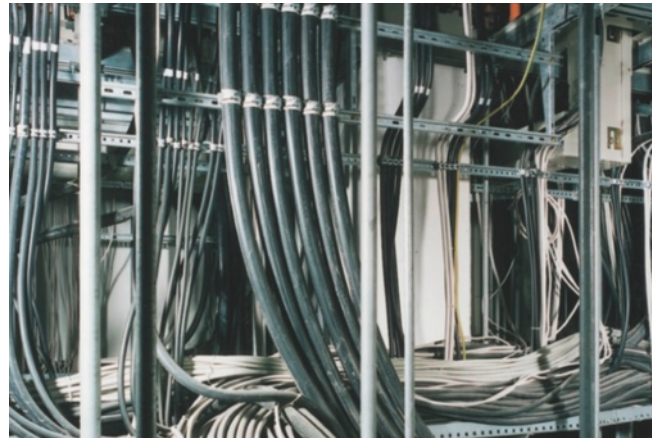
High fire load with cables
