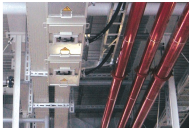
Low fire load with busbar trunking system
