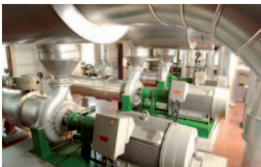
Hot water pumps in the heating system of a car manufacturer
