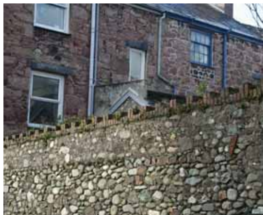
Random rubble to the rear of Segontium Terrace, and river stones in the boundary wall.
