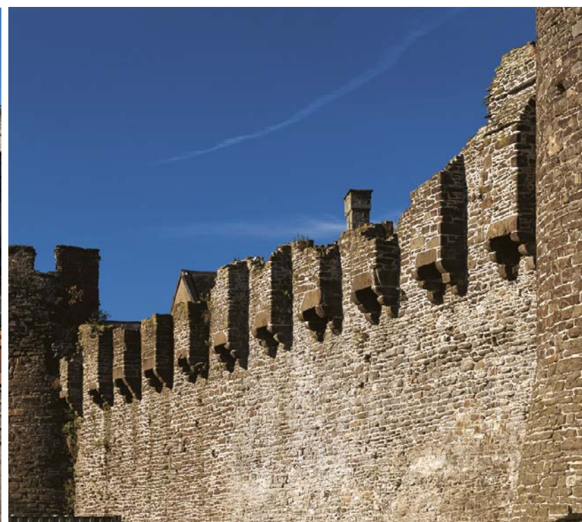
Medieval latrines projecting out over the town wall probably served the offices of medieval administrators located in a building on a site close to Rosehill Street.
