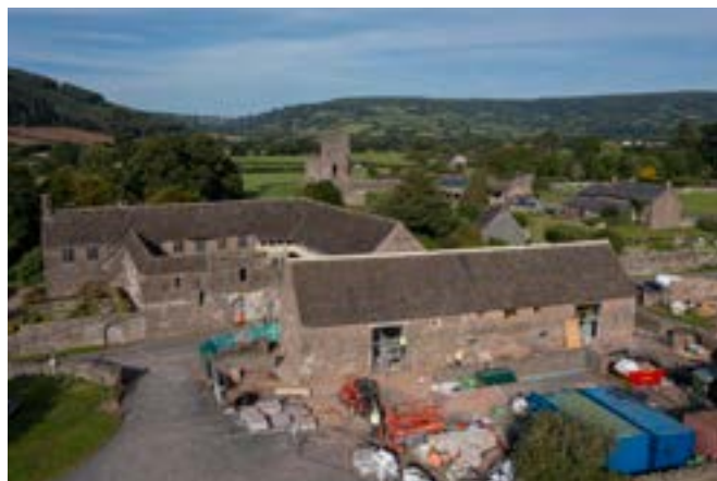
Top: A view of the ongoing work at Caernarfon Castle, Gwynedd, to install a rooftop deck and reinstate the floors in the King's Gate to enhance the visitor experience.
