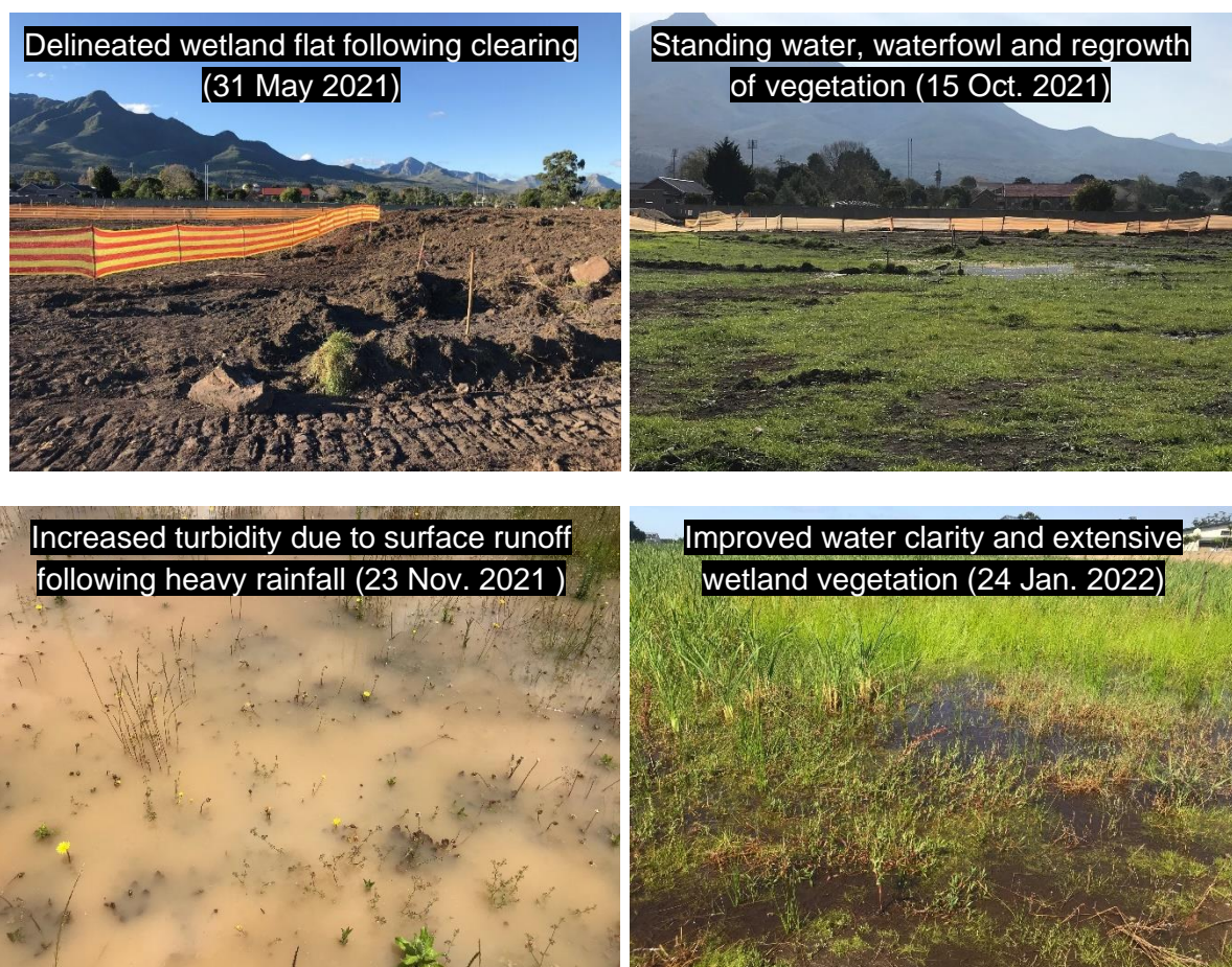
Figure 3. Photo of the wetland flat immediately after it was excavated, partially infilled and delineated (top left), approximately 3 months following removal of the infill material and cessation of work in the area (top right), water quality following heavy rainfall on 22/11/21 (bottom left), and following extensive regrowth of vegetation and good rains (bottom right).
