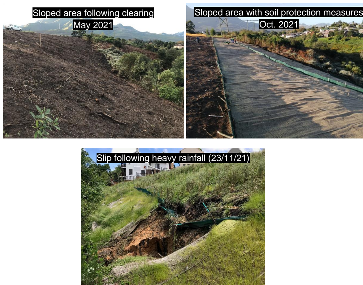
Figure 2. Photo of the area where riparian vegetation was cleared (left) subsequently stabilised with soil erosion control measures (right), and where a slip occurred following heavy rainfall on 22 November 2021 (below).
