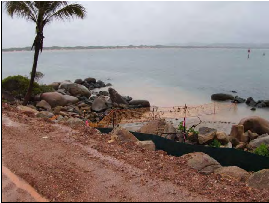
Figure 3.30 Sediment run-off from an Endeavour River waterfront construction site
