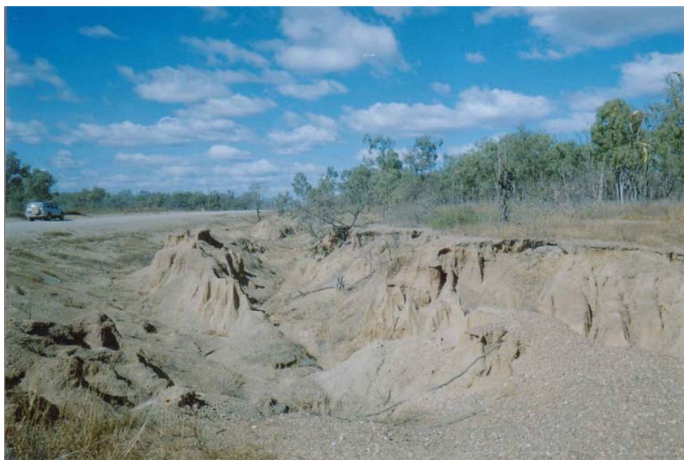
Gully erosion on the road from Lakeland to Laura
