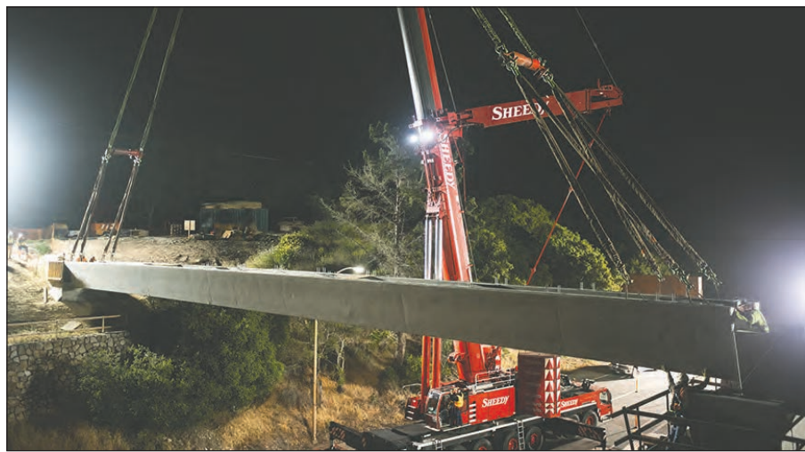
Construction crews Tuesday night installed these tub girders over Highway 68 in Monterey for a pipeline that will deliver drinking water to the Monterey Peninsula.
