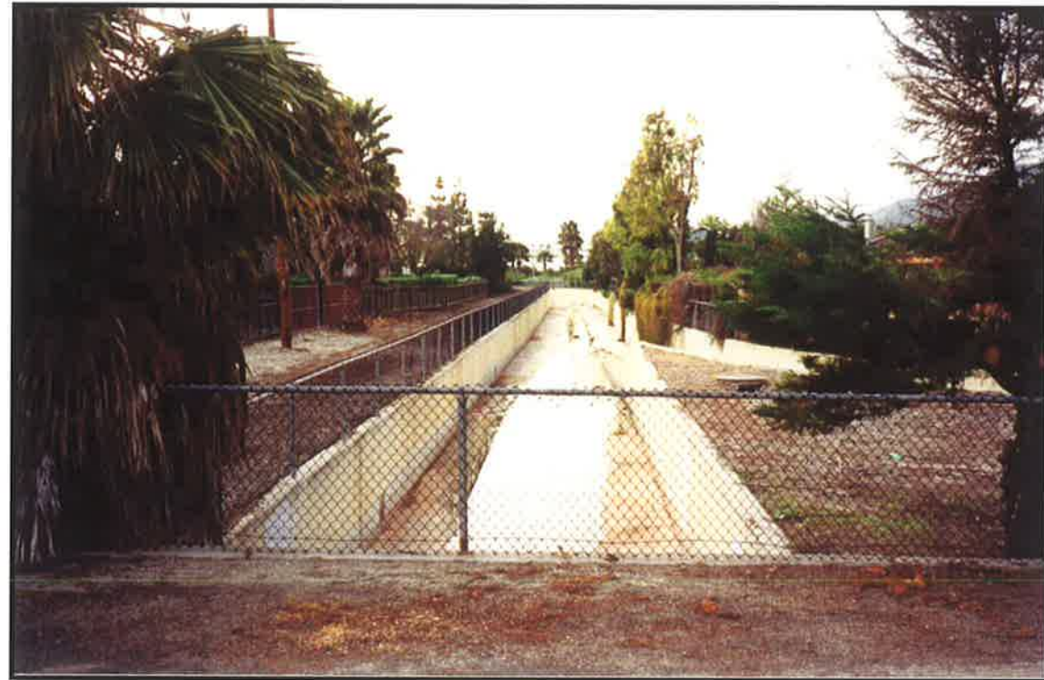
Looking west along the Main Channel of Franklin Creek, from near the Foothill Rd. / Linden Ave. intersection. The West Branch of Franklin Creek enters the Main Channel in the mid-ground of the photograph. These formerly natural creeks have been converted to concrete box channels.
