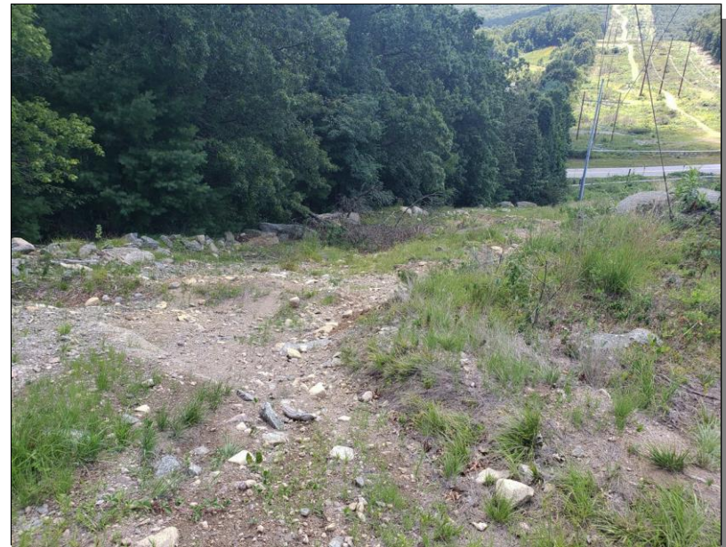
Photo 30: Runoff has already caused substantial erosion on the steep south-facing hill below the new pads on the hilltop. It was worsened by cutting multiple red cedars that had anchored the hillside soil. 8-16-19.
