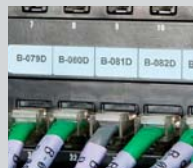
Patch panel and terminal block ID
