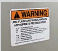
Arc Flash and safety labels
