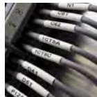
Wire and cable labeling
