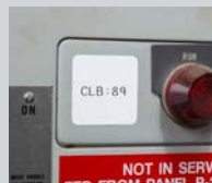
Asset and equipment ID
