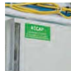
Control panel labeling
