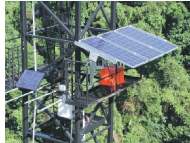
Fig. 67. Solar panels permanently attached to the crane tower help power auxiliary equipment (photo Michael Cermak).
