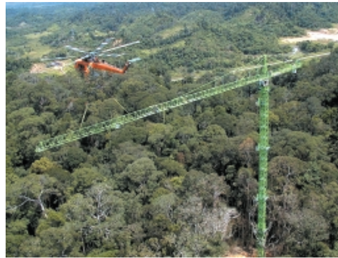
Fig. 77. The end section of the Lambir Canopy Crane jib being lowered into position (photo Tohru Nakashizuka).
