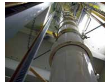
The renovated 6-inch glass distillation column in our Unit Operations Lab
